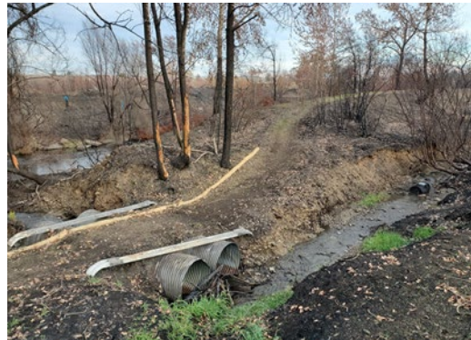
Hoop trap at Elk Ck double culvert
